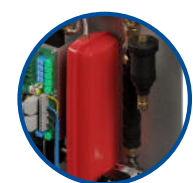
CH expansion vessel
